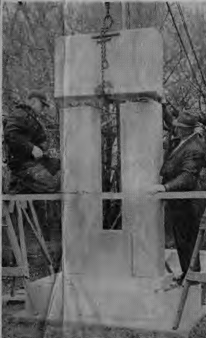
LOWERING THE LAST SECTION on the veteran's memorial are workmen from the Simpson Granite Works of Libertyville. The job took seven hours to complete. Located at the southwest corner of Heritage Park, the $3,000 gray granite memorial is dedicated to all Wheeling men who have served in the wars.
